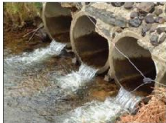
Unacceptable culverting practice. These pipes are totally impassable to fish.
