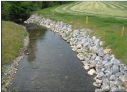
The boulders in these bank protection works are not large enough, not sunken below stream bed level and likely to be undercut and dislodged in a storm event.
