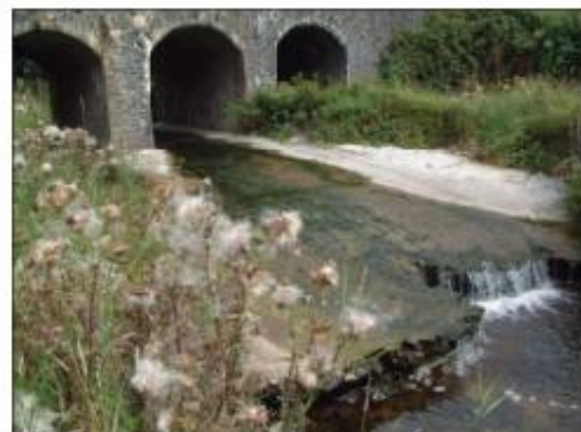
Apron/scour slab inaccessible on its downstream end to fish life because of the extent of perching and impassable due to a combination of excessive water velocity and lack of water depth across its surface.
