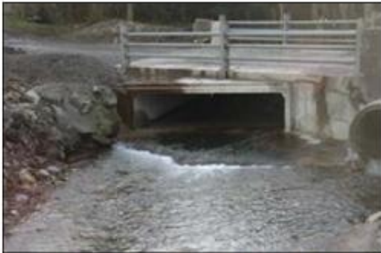
Box culvert positioned at incorrect level. Upstream fish passage is made difficult. Culvert invert should be 500 mm. below existing bed level and back filled with clean gravel to match the existing stream profile.
