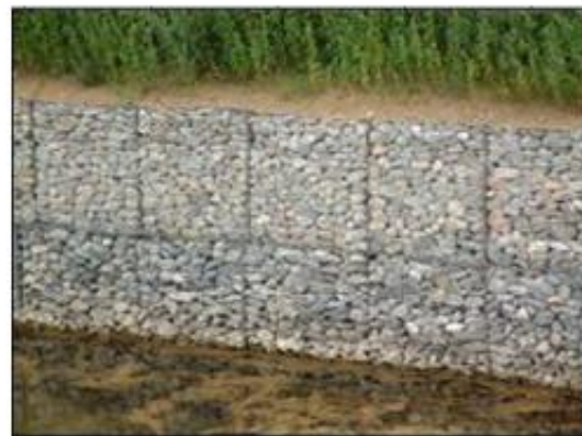
Visually unsightly stone filled gabion baskets.
