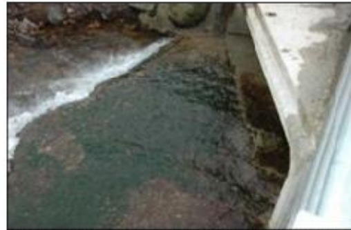
The smooth concrete finish is totally unsuitable for fish passage.
