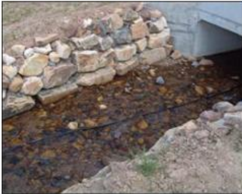
An embedded box culvert sized to match existing stream profile.
