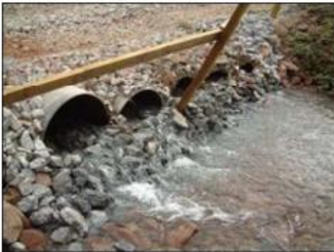
Temporary crossing impassable to fish life.
