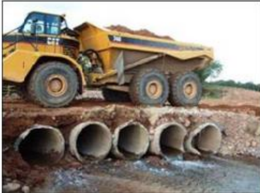
The same temporary crossing location as shown on the previous page, but with a laden dumper dislodging and causing loss of cover material to waters.
